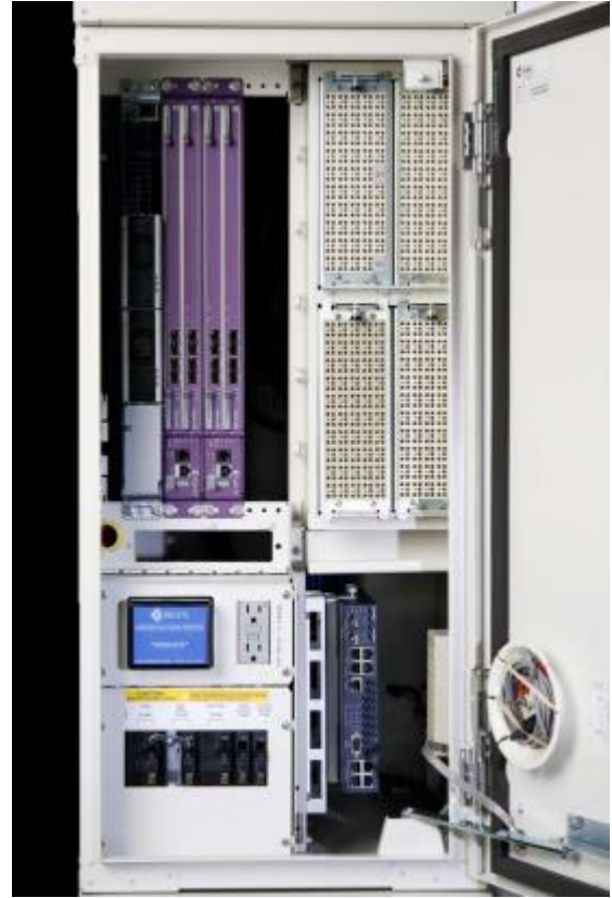
ODC-100 w/ 192 VDSL2 Combo Ports and Copper Transport
