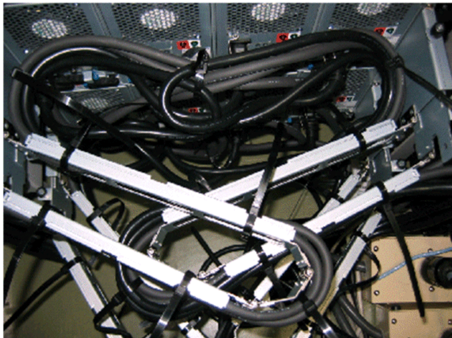
Figure 5-36: ENC Cable Routing on High-density Expansion Unit
