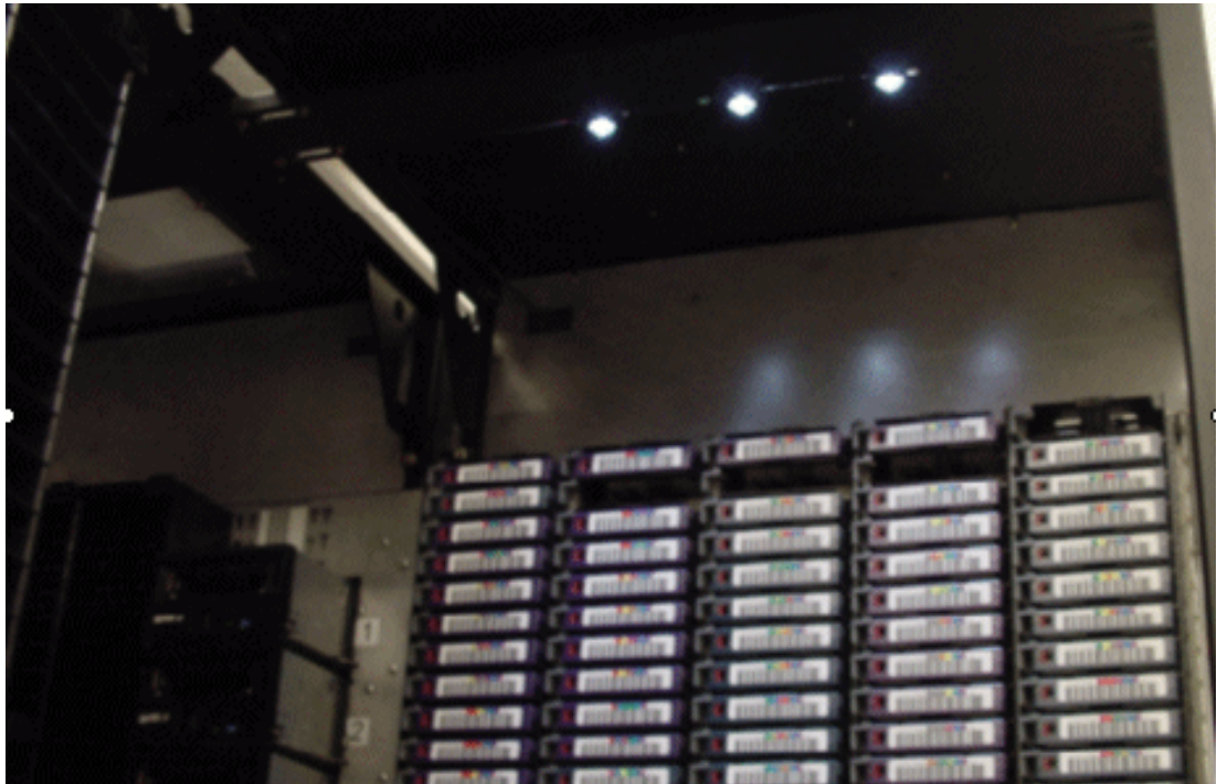
Figure 12-8 internal LED lighting
