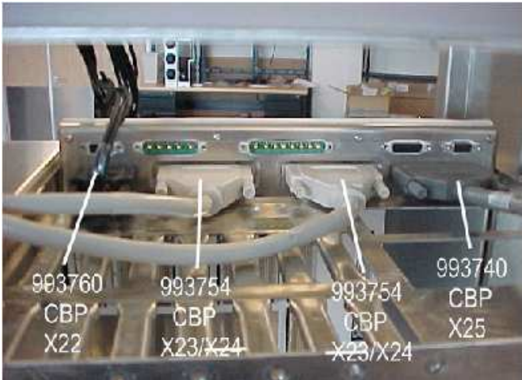
Figure 1. Common backplane bottom row cabling
