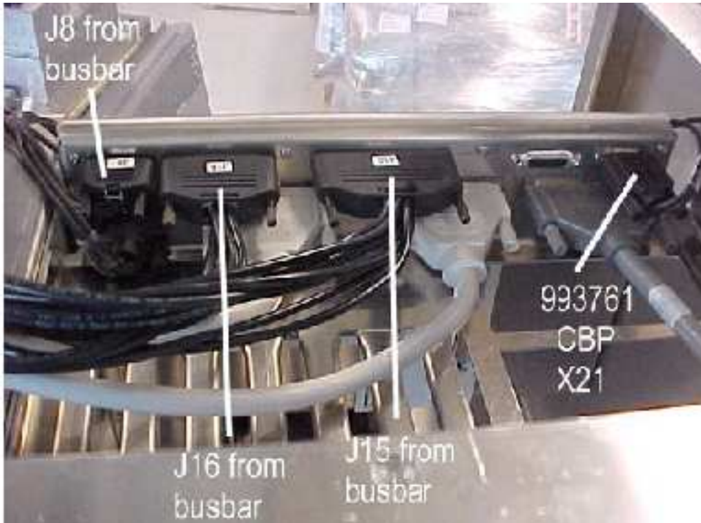
Figure 2. Common backplane upper row cabling
