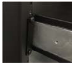
Figure 1b: Rack installation
