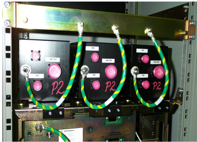
Figure 52 Finished Horizontal Mount Assembly – Rear View
