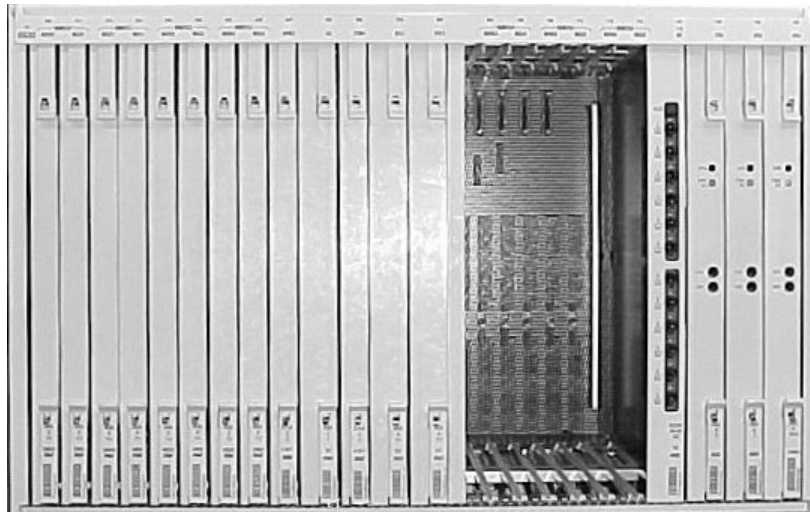
Figure 1-18. DS3U Circuit Pack Positions (Photo similar to HDS3U)
