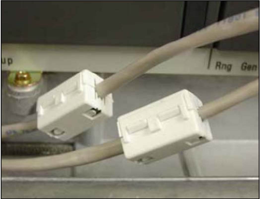
Figure 154 Attached Ethernet patch cable ferrite beads
