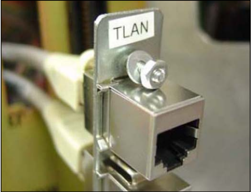
Figure 152 TLAN connection on Ethernet port coupler
