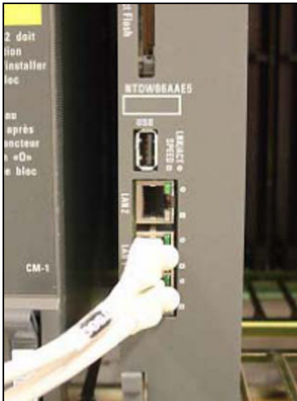
Figure 106 TLAN connection on faceplate
