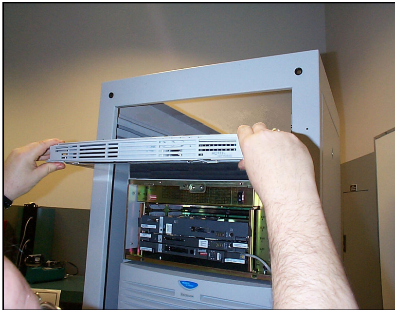
Figure 39 Rack-mounting the ISP1100 Signaling Server
