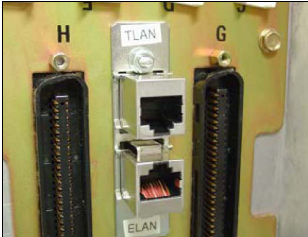
Figure 31 Installed Ethernet port adapter plate
