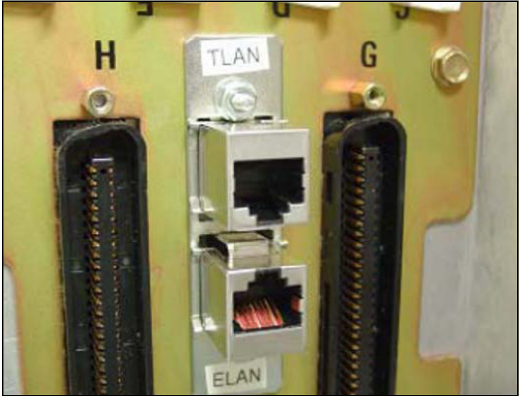
Figure 21 Installed Ethernet port adapter plate
