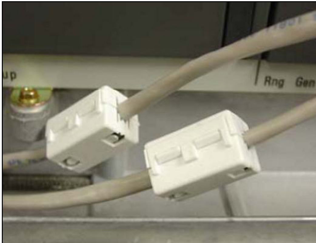
Figure 39 Attached Ethernet patch cable ferrite beads
