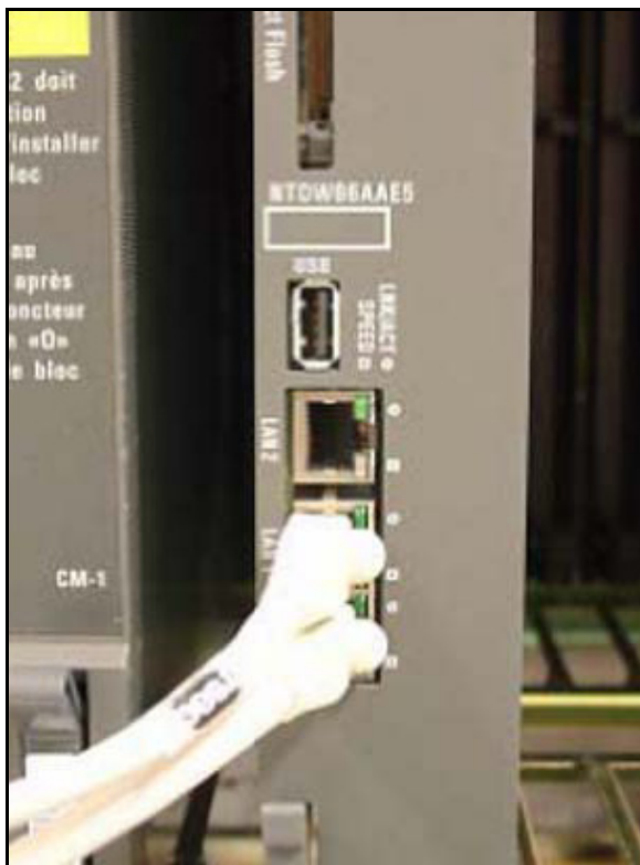
Figure 36 TLAN connection on faceplate
