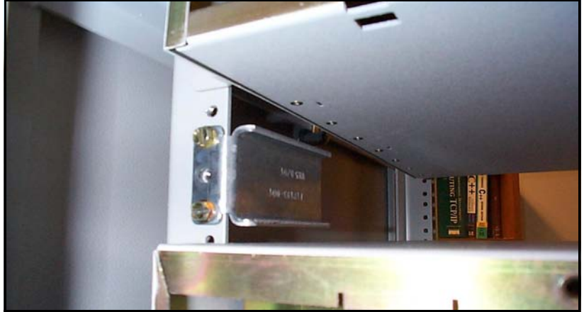
Figure 55 Installed rack-mount bracket
