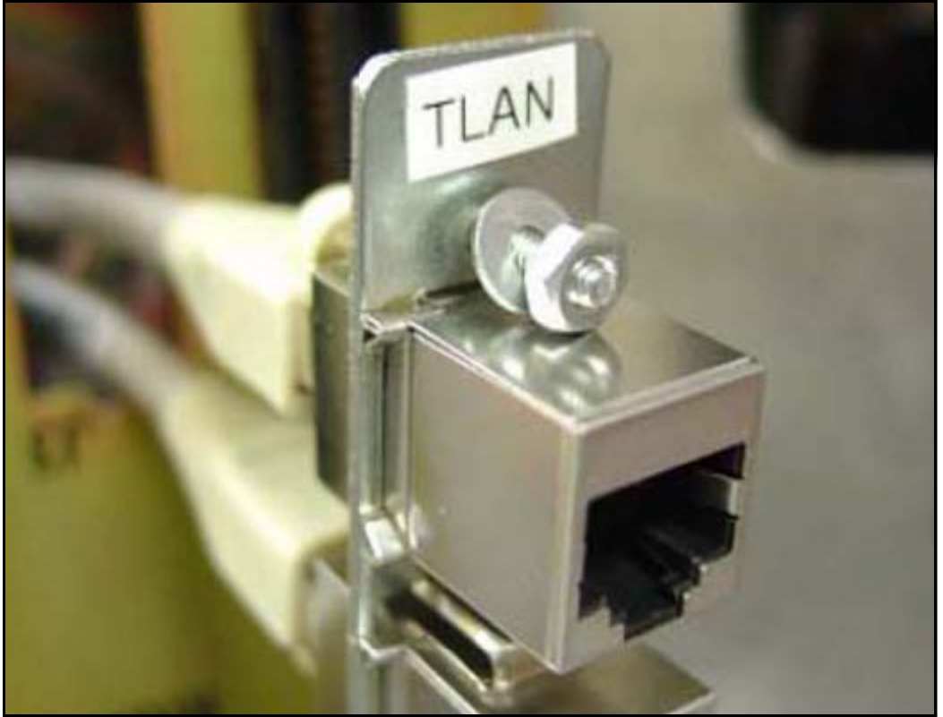
Figure 49 TLAN connection on Ethernet port coupler
