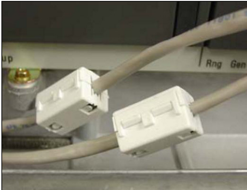
Figure 50 Attached Ethernet patch cable ferrite beads
