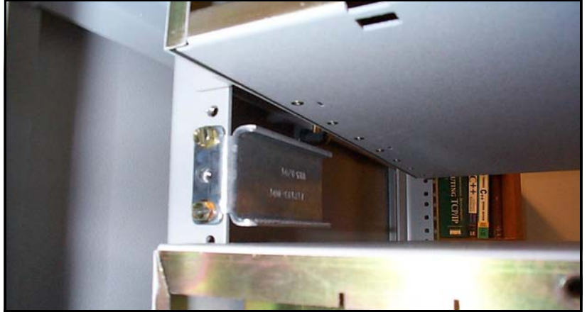
Figure 56 Installed rack-mount bracket
