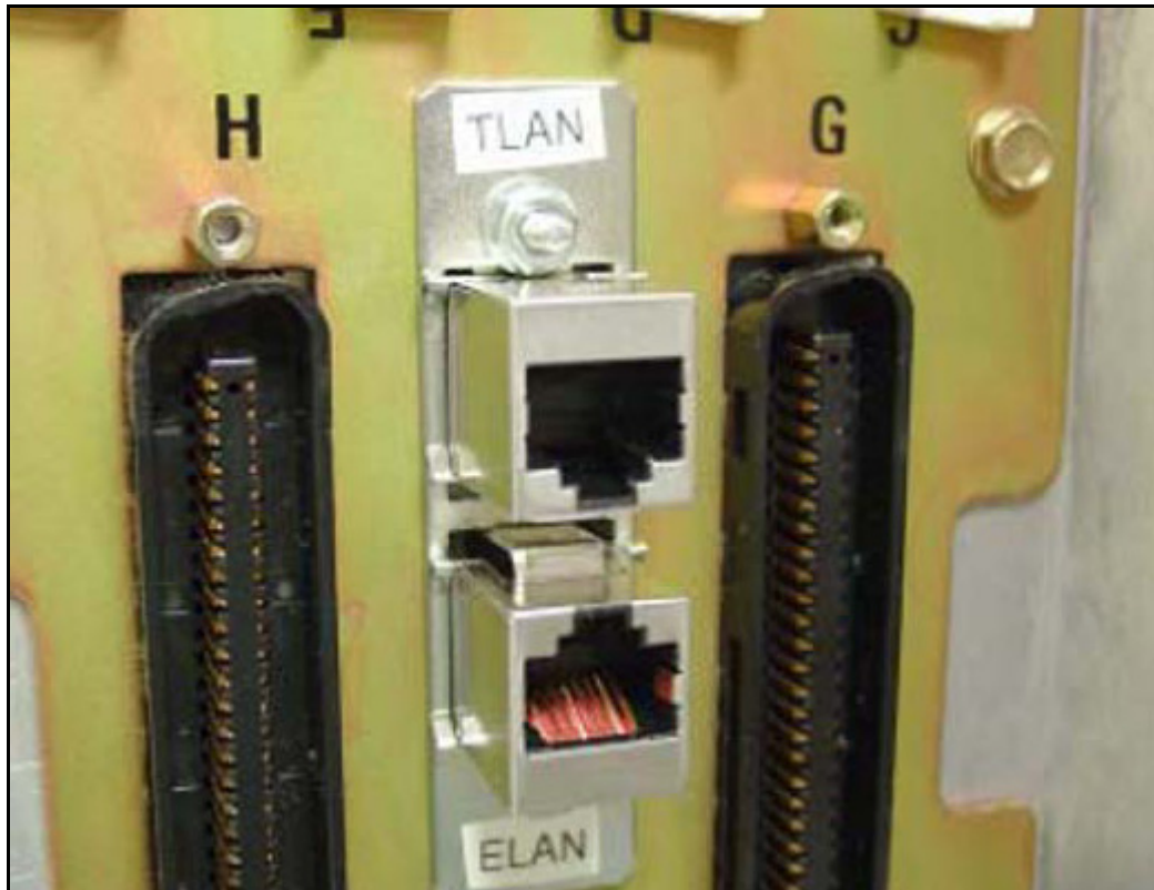
Figure 40 Installed Ethernet port adapter plate
