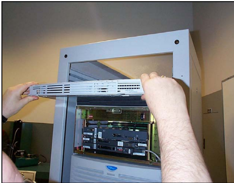
Figure 41 Rack-mounting the ISP1100 Signaling Server
