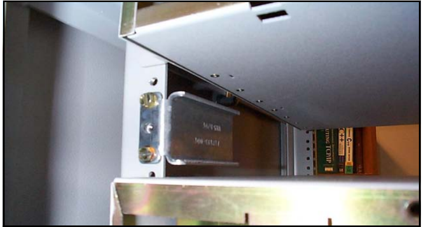
Figure 40 Installed rack-mount bracket
