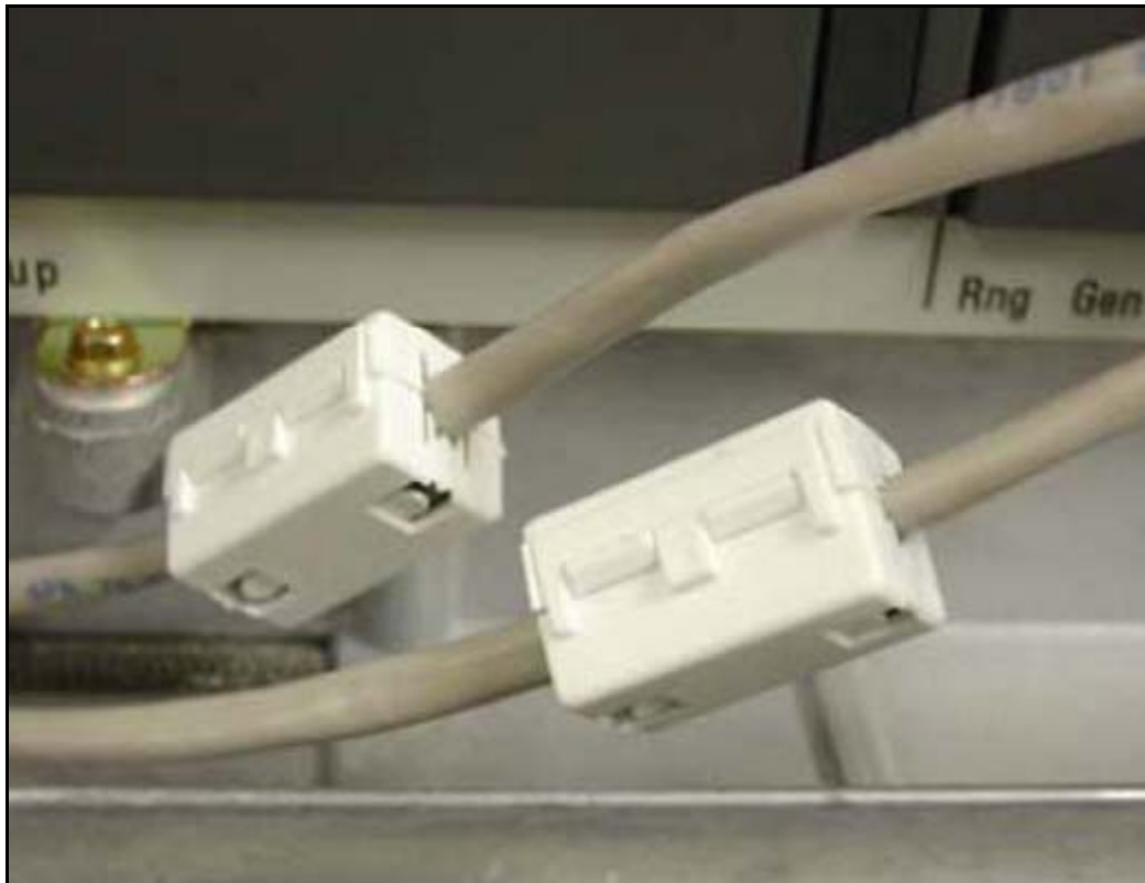
Figure 53 Attached Ethernet patch cable ferrite beads
