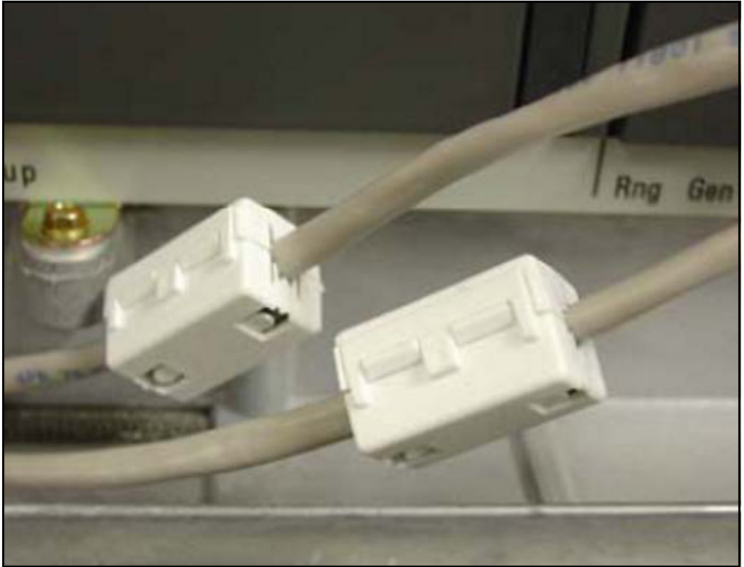
Figure 50 Attached Ethernet patch cable ferrite beads
