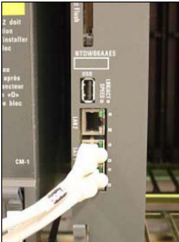
Figure 47 TLAN connection on faceplate
