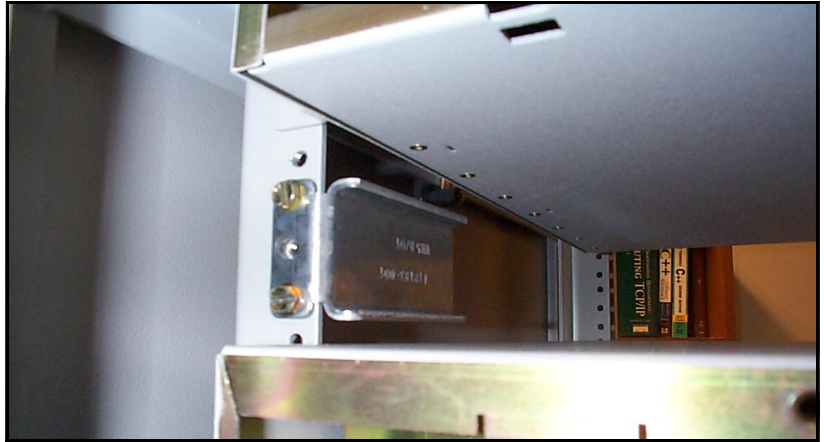
Figure 56 Installed rack-mount bracket
